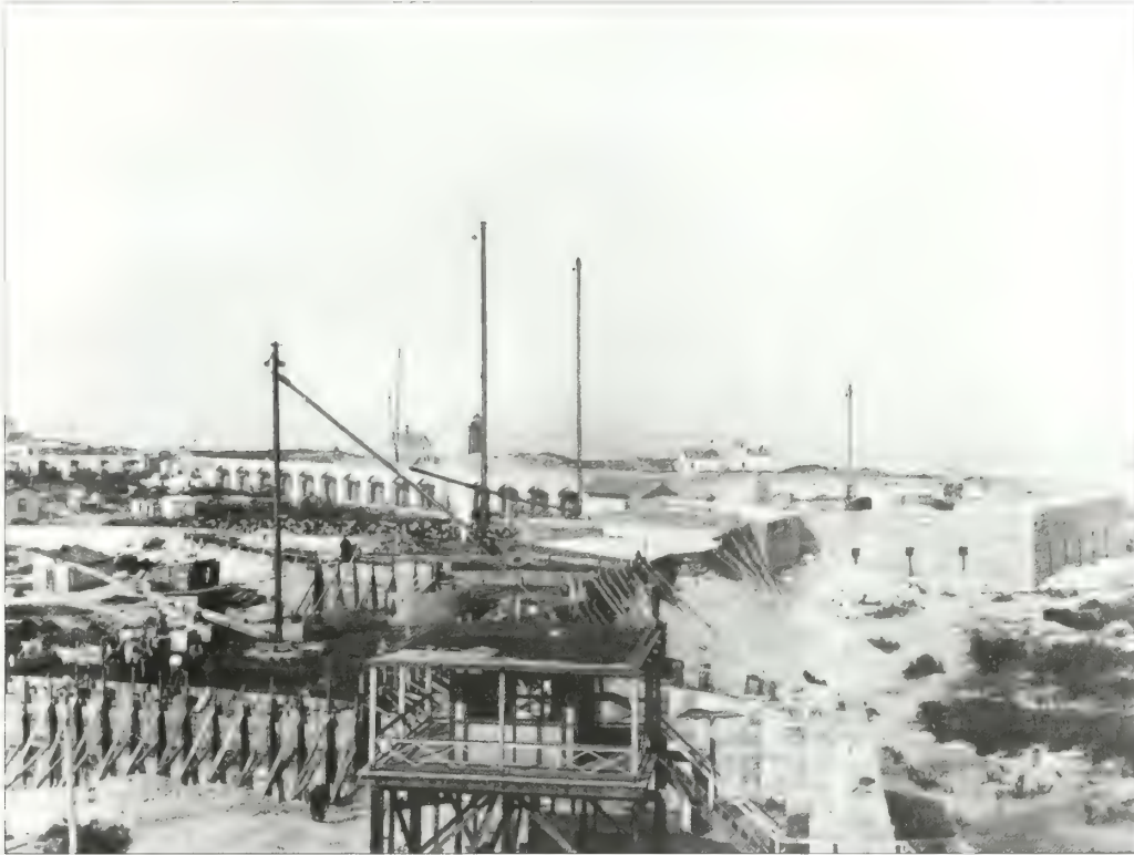
Figure 5.54. Construction of Nine Gun Battery, 1897. The concrete battery structure was built over a Civil War-era granite block fort. The fort's bastions can be seen in the image as the forming of the battery occurs over the fort's eastern wall (GATE 7880).
